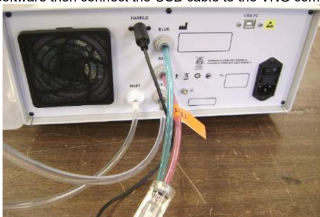
Figure 3 Tubes and Electrical Connection
